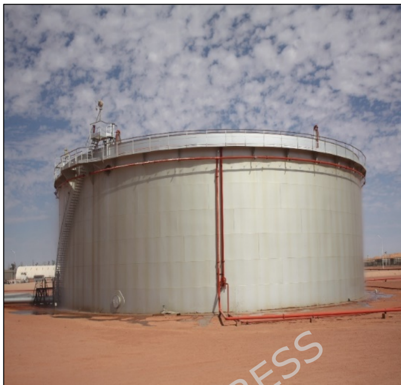
Figure 5. Oil storage tank A12.
