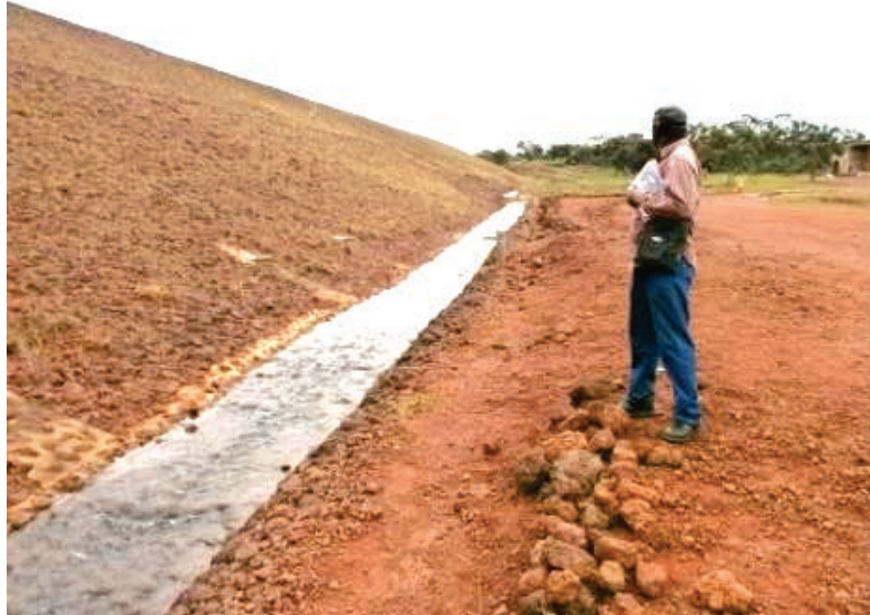
Fig. 8. Leakage flows along the dam toe
