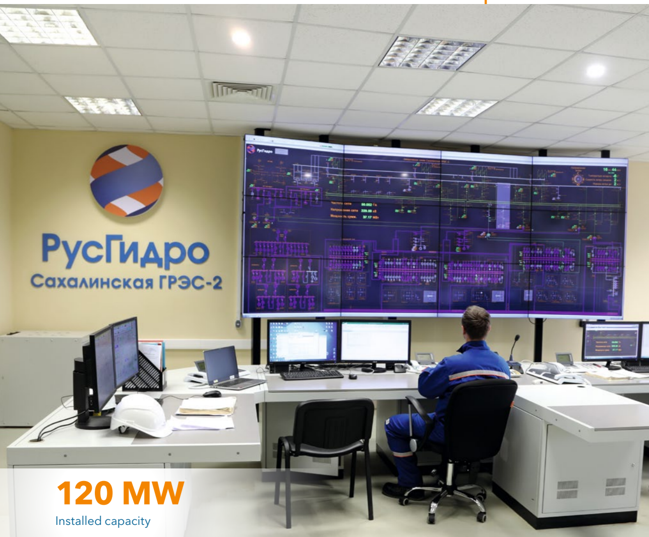
Sakhalinskaya GRES-2, Sakhalin
